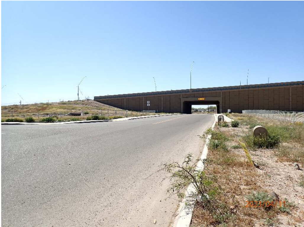
Davis Avenue looking south from the southeast corner of the subject property.
